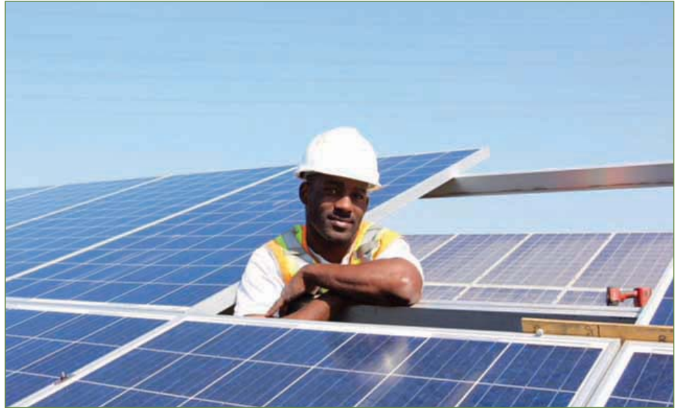
MCE is adding contracts with PV solar developers and developing its own 10.5 megawatt facility in Richmond.
